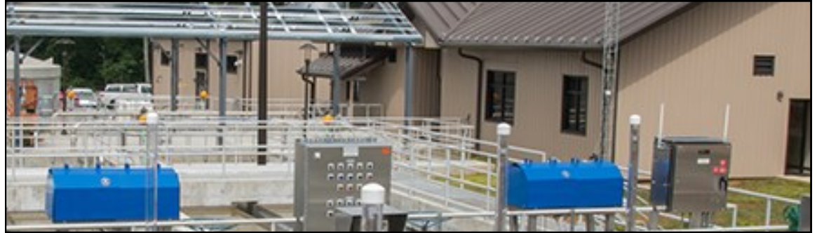
City of Roswell's Water Plant
