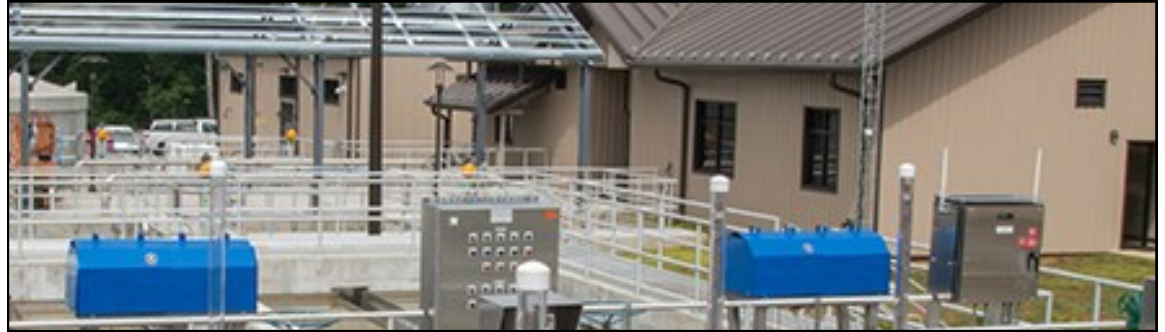
City of Roswell's Water Plant
