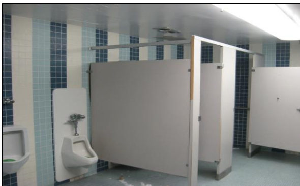
Civic Center restrooms in need of renovation
