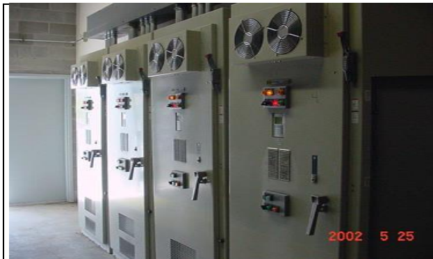
Current variable frequency drive equipment at plant
