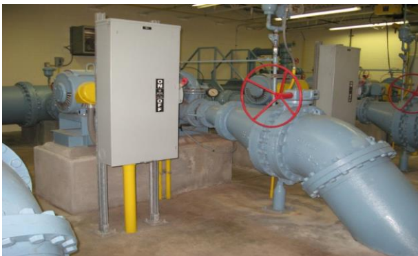
Equipment at Crossroads Booster Station
